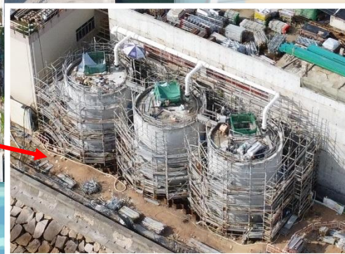
Works for Sludge Holding Tanks in Progress 污泥儲存缸工程進行中
